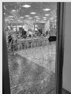
Kibbutz Nir Oz – Entrance doors to the dining hall. Kibbutz still has no residents; no repairs since October 7th.
